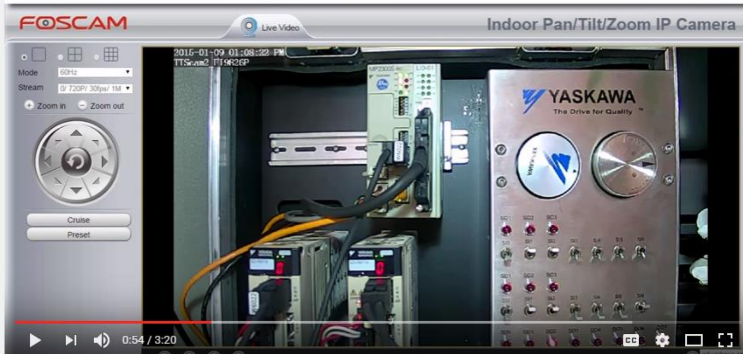
Reset MPiec Controller to Default in MotionWorks IEC
